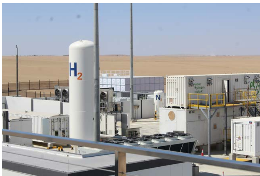
A view of the core hydrogen production and storage facilities at Cleanergy Green Hydrogen Plant and Refuelling Station Solutions Namibia
